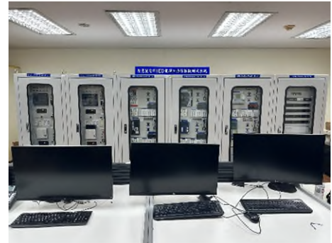
智慧變電所 IED 電驛互操作性模擬測試系統 Smart Substation IED Station Interoperability Simulation Test System
