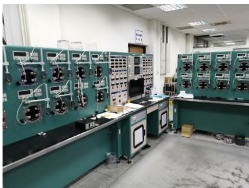
電度表修校自動化設備 Watt-hour Meter Repair Automation Equipment
