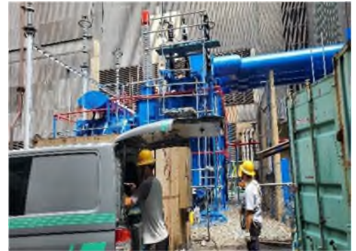
變壓器絕緣試驗 Transformer Insulation Test
