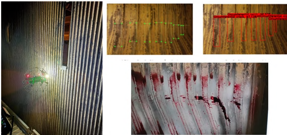
鍋爐無人機巡檢、影像辨識與破損分析 Drone inspection, image recognition and failure analysis
