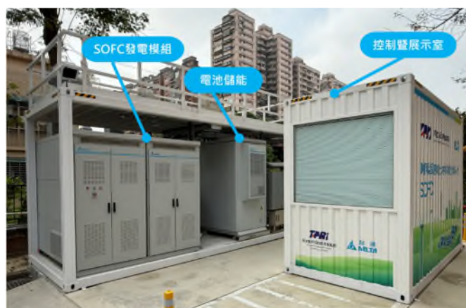
併網型固態氧化物燃料電池發電系統(SOFC) Grid-connected Solid Oxide Fuel Cell (SOFC) Power Generation System
