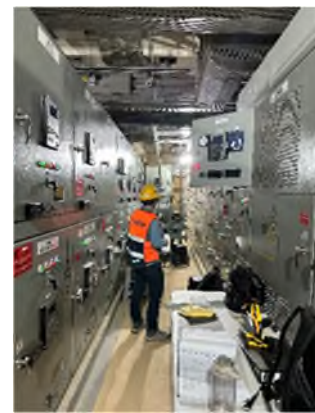
發電廠變電所 IED 功能特性驗 IED Functionality Verification in Power Plants and Substations
