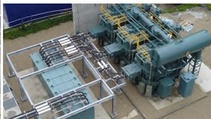
大容量短路試驗室 Large Capacity Short Circuit Lab
