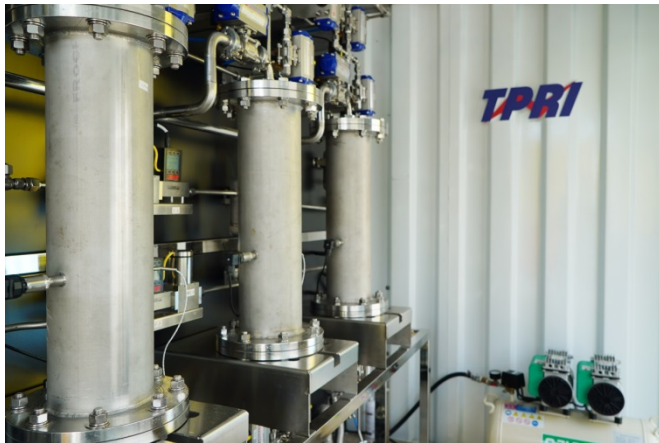
Fig.5 The main facility of 3-bed pressure swing adsorption CO 2 separation.
