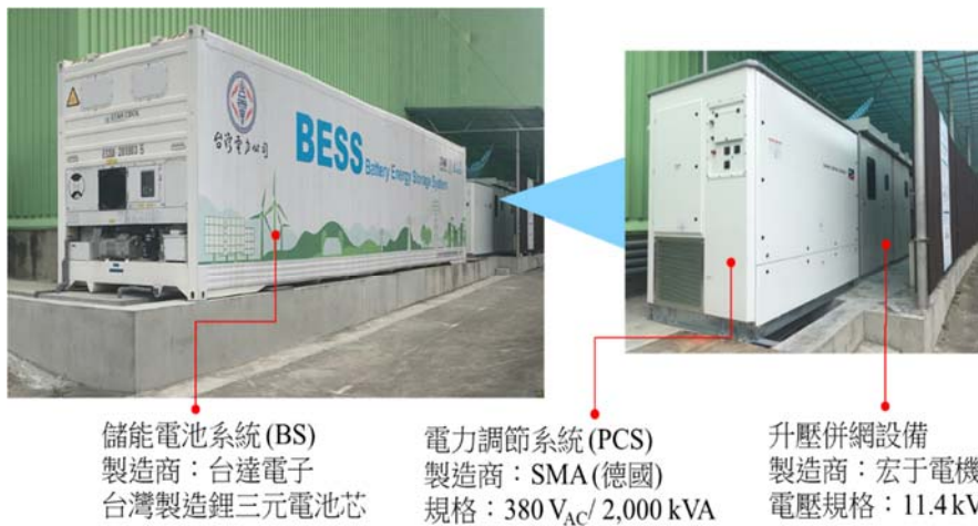
Figure 2 Photographs of 1MW/1.5MWh containerized lithium-ion battery energy storage system
