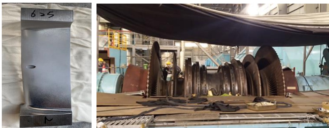
Fig. 3 Photo of the welded test specimen (left) and the blades to be repaired on the steam turbine rotor (right).
