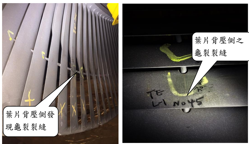
Fig. 1 Photo of the suction side of the low-pressure turbine blades (left) and the location of its crack(right).
