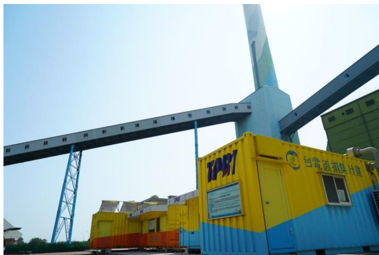
Figure 4: Container Equipment of VPSA (Two 20-foot Yellow and Blue Containers) (Photographed by TPRI)
