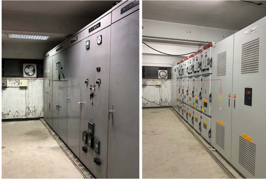
Figure 1 Before (left) and after (right) renovation of the high-voltage substation at FDSO
