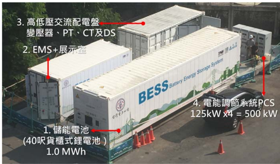
Figure 3 The 500 kW/1MWh lithium-ion container energy storage system
