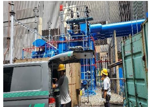
變壓器絕緣試驗 Transformer Insulation Test
