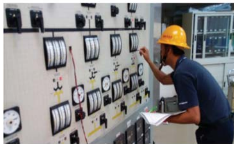
Period calibration of monitoring devices in power plants and distribution stations
